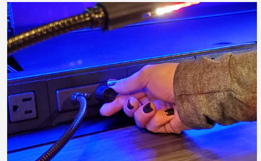
Single-point dimmer control is within the operator's primary reach zone.
